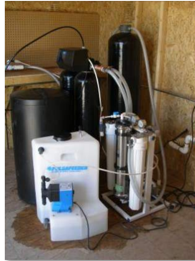
Reverse Osmosis System Used to Remove Arsenic from Drinking Water
