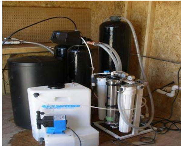
Example of a reverse osmosis system installed in the San Antonio del Desierto Mobile Home Park by Pueblo Unido Community Development Corporation for the STAT Project.
